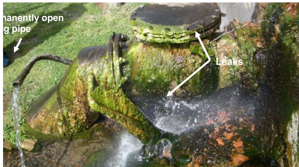
Figure 0.6 Damaged pressure pipe in the water intake.
