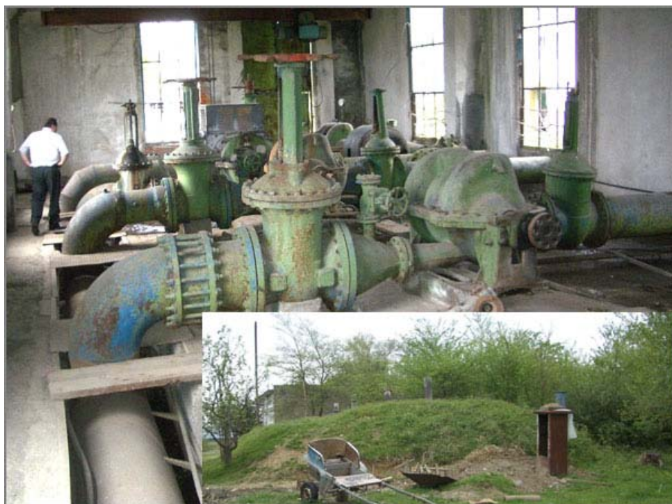
Figure 0.2 Second lift pumping station and clear water reservoir (CWR) V=500 m 3 .
