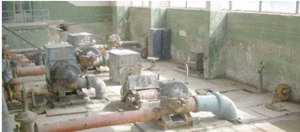
Figure 0.2 The second lift pumping station. Pump D 1250-125.
