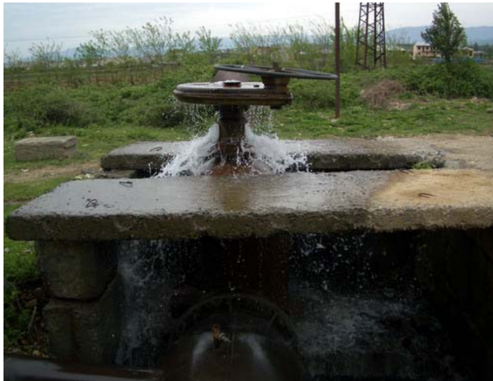
Figure 0.2 Leaking valve (D800mm) on the pressure water main on second lift pumping station, Kutaisi.
