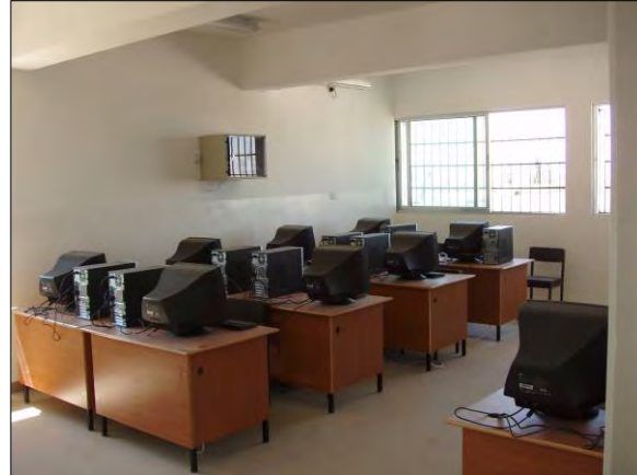
Exhibit 4 A new computer lab at Salah Al-Din School cannot be used because electrical outlets are in the wrong location.
