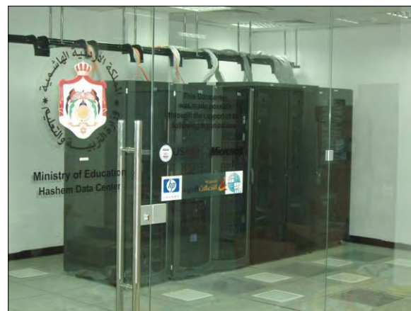
Exhibit 2 The Ministry of Education data center co-located at the Jordan Telecom Hashem Data Center.
