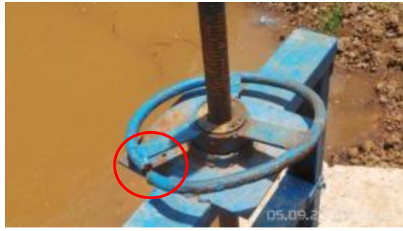
figure 15d: Mechanism to close and open the sluice gate is damaged, it is believed that the rust constantly increases the force needed to open and close the sluice gate, until its breaks.
