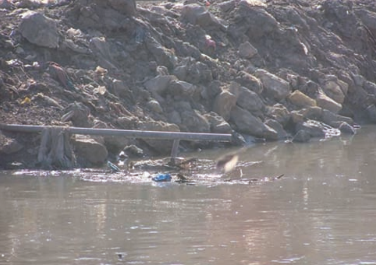
Pipe connected to canal
