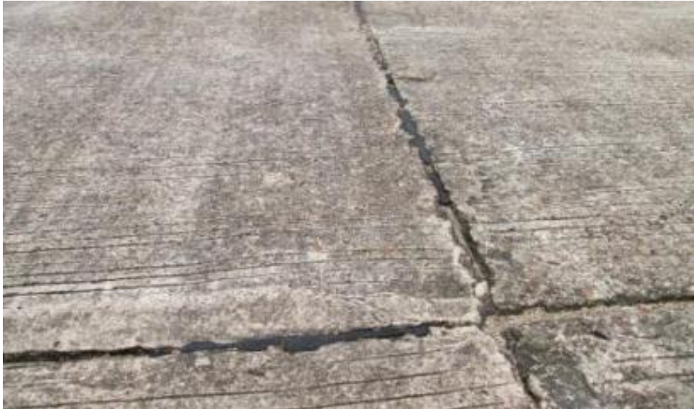
<Photo 4-6> Paved Runway before the Rehabilitation (Repaired during the Recovery Development Period)
