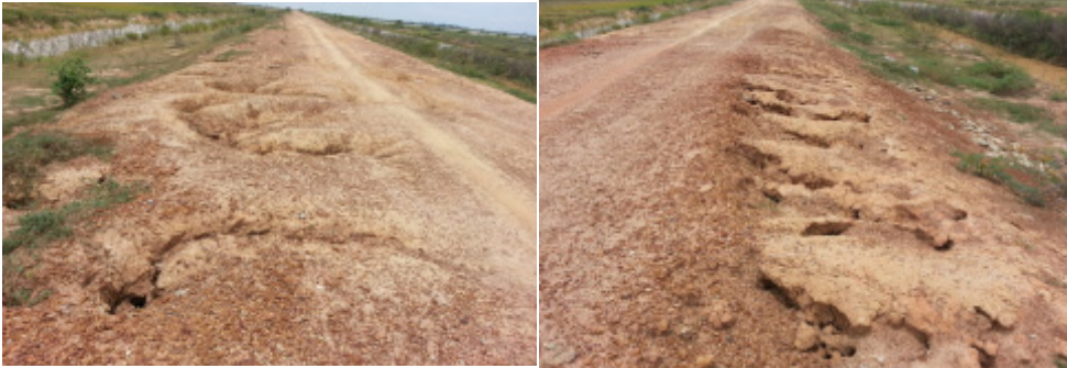
[Figure 8] Damage to Dike Road After Flood
