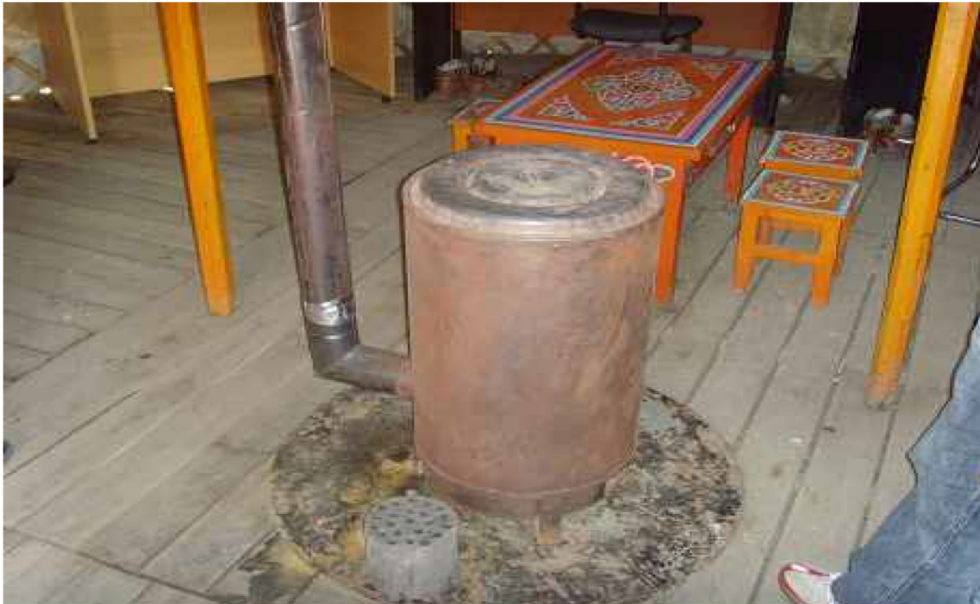
<Figure 3-8 Yeontan stove installed in Gerr>
