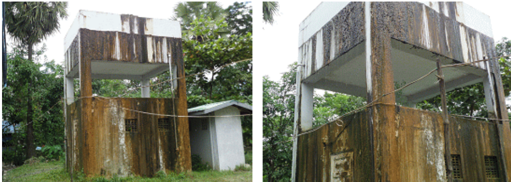
<Serious water leakage in a tank - Kha Young village>
