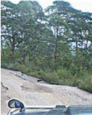
A road with surface damage
