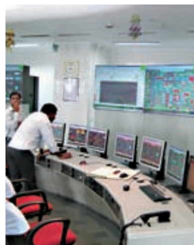
Central Control Room
