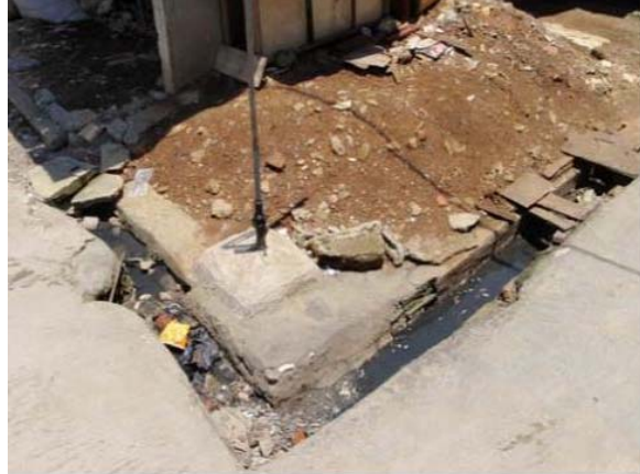
Photo A7.15: Clogged drain in the KIP area
