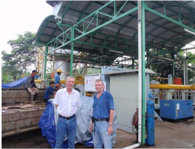
Photo A7.11: New Clean Development Mechanism in Sumur Batu final dumpsite
