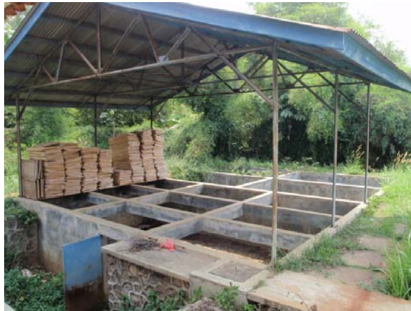
Photo A7.5: Pilot wastewater treatment plant (300 households)
