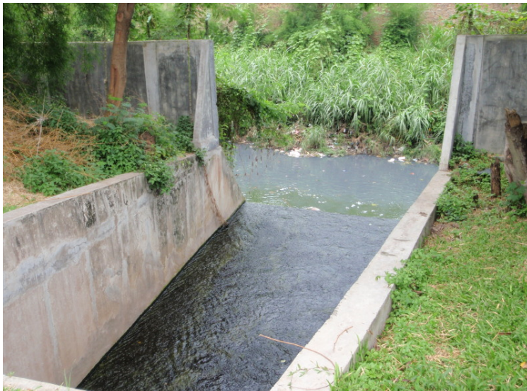
Photo A7.2: Discharge of treated water, which is cleaner than the river water
