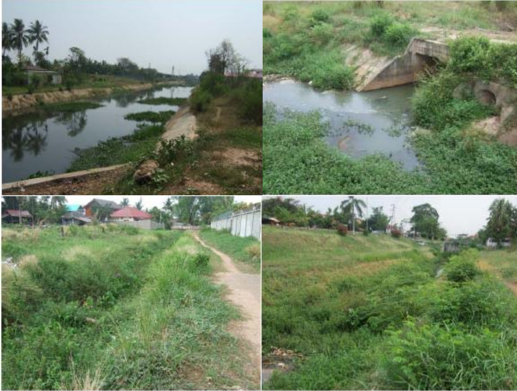
Photo A7.12: Drainage full of vegetation needs maintenance
