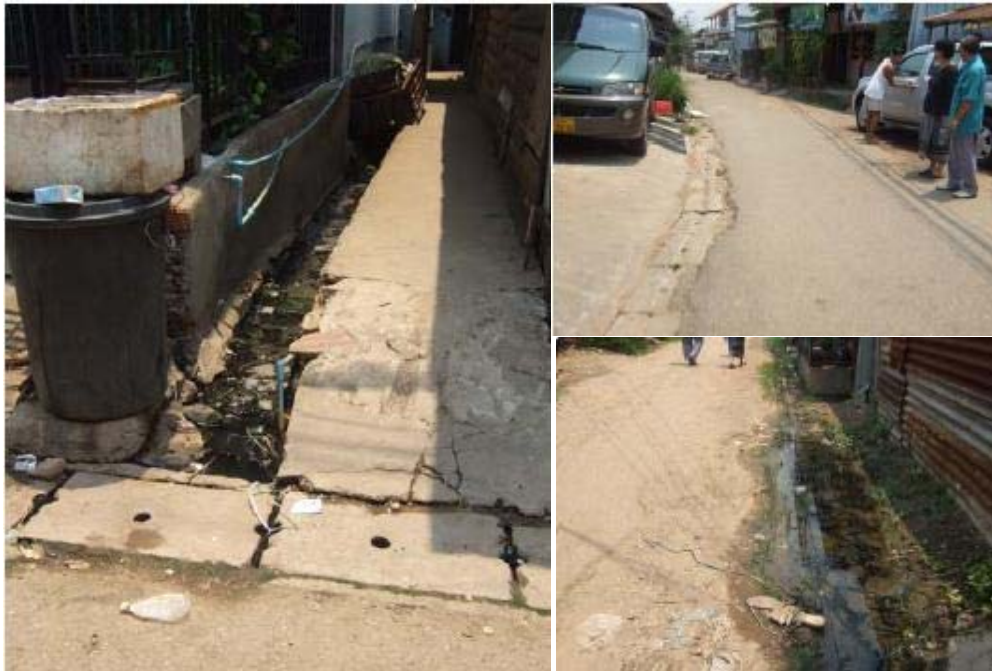
Photo A7.11: Village area improvement road at Phonsavanh Neua village; the drainage system has problems
