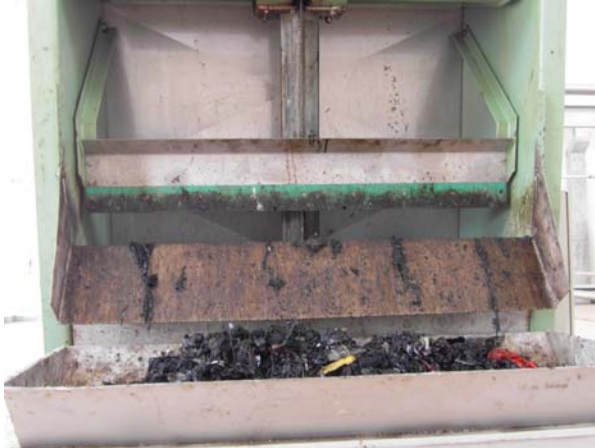
Photograph A4.1: Screening Discharge at Inlet
