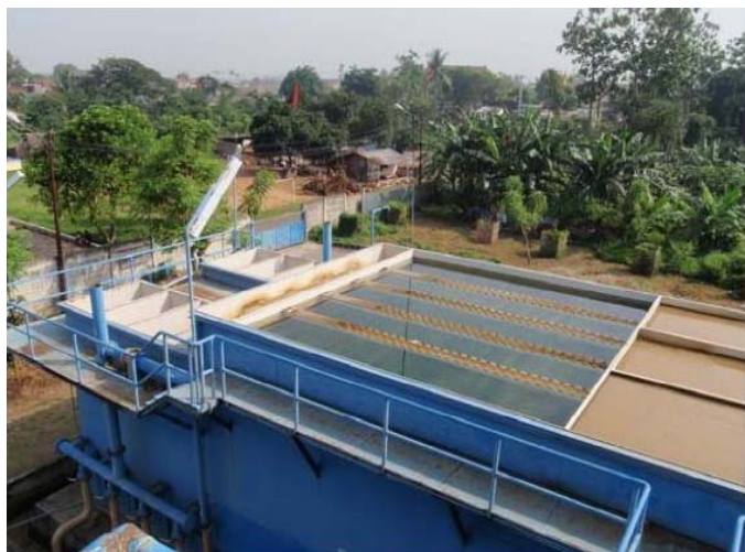
Bajuceper Water Treatment Plant
