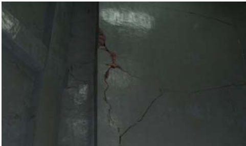
These are the cracks on the walls of UNAND in Padang caused by frequent earthquakes.
