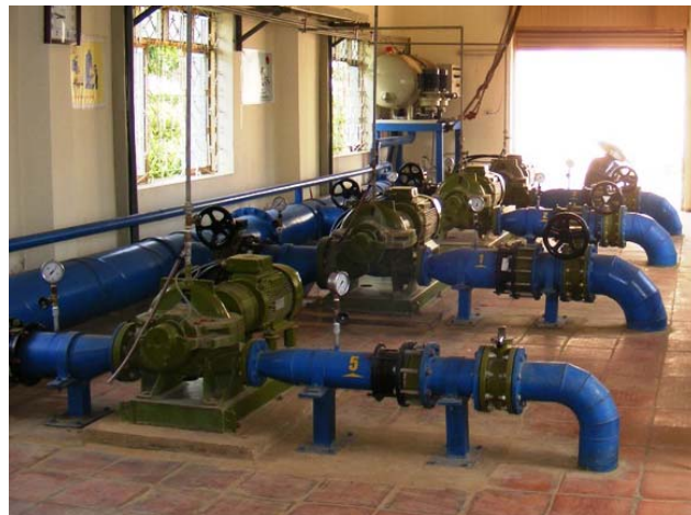
Figure A4.2: Inside Tuyen Quang Pumping Station
