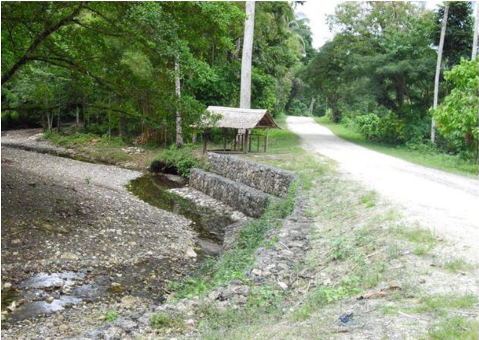
Photo A9.8: Gabion treatment of creek bank to protect unsealed rural road (Malaita South)
