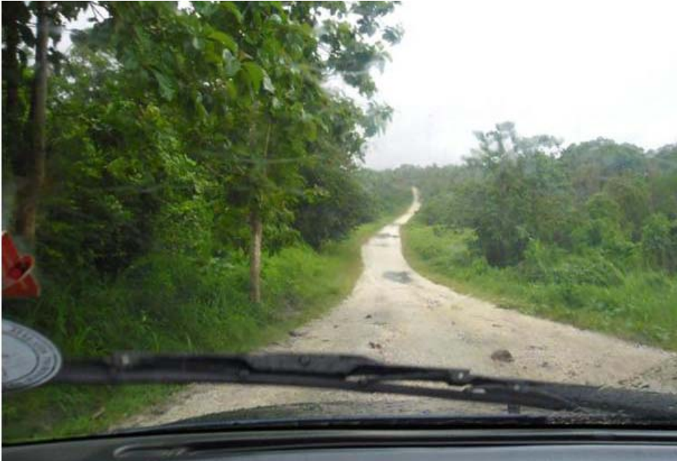
Photo A9.7: Unsealed rural road showing maintenance patching (south of Loudulou Bridge)
