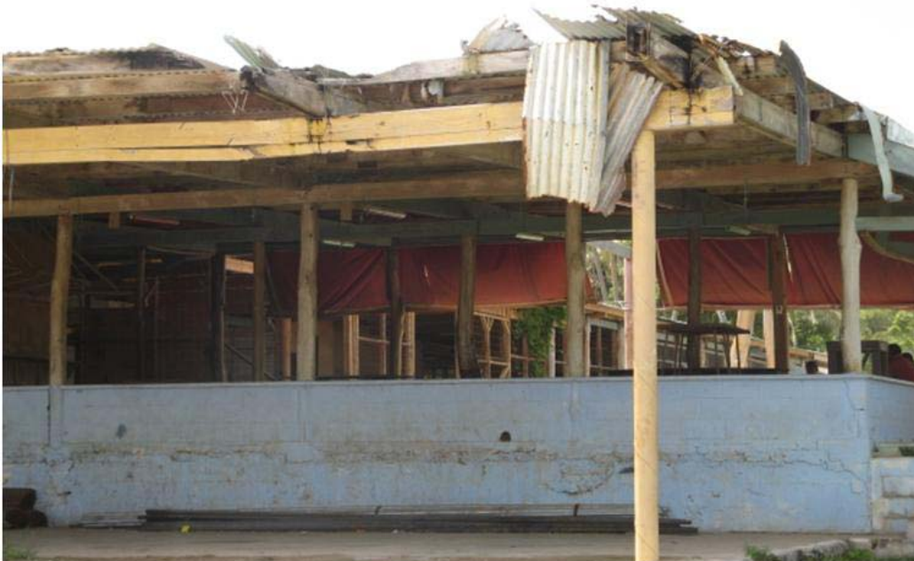
Photo A9.18: Cyclone damage not yet cleared away in Atutuki (not under ADB emergency loan). This shows sample of damage.
